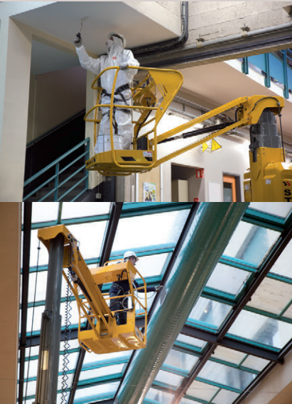
INDOOR FINISHINGS (electrical, lighting, plumbing, painting, HVAC, piping, fire detection systems, etc.)
